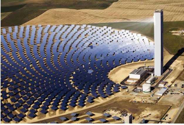
Figure 2. Heliostat solar power plant
