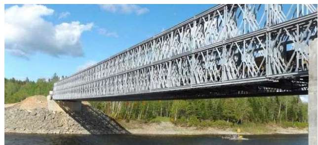
Figure 9. The bridge was reconstructed by using a steel structure to withstand climate change impacts in the North of Mozambique [18]
